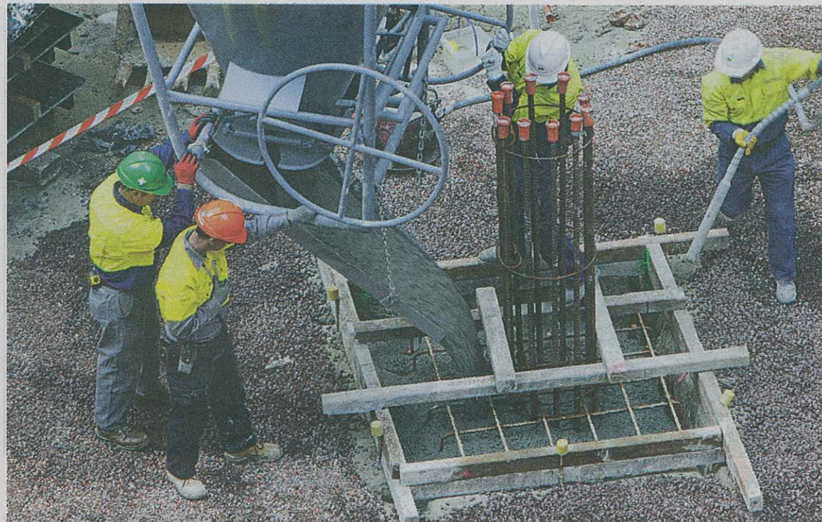
Thin on the ground . . . commercial construction starts are expected to decline 50 per cent this year.
